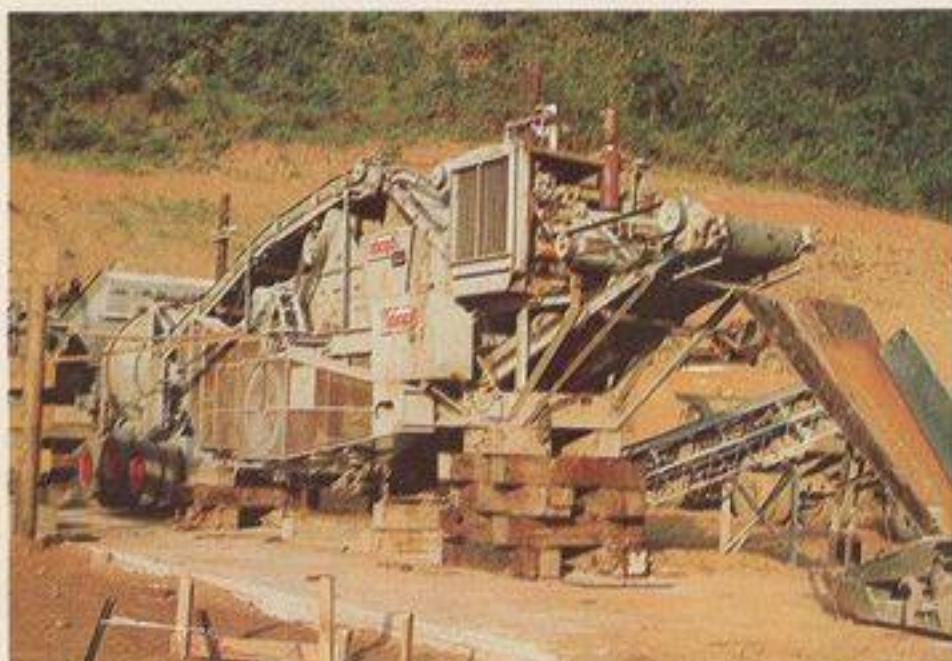
The SeaBees operate six crusher plants in Vietnam. This unit, one of the largest in the SeaBee inventory, is run by MCB-9, and is powered by Detroit Diesels.
