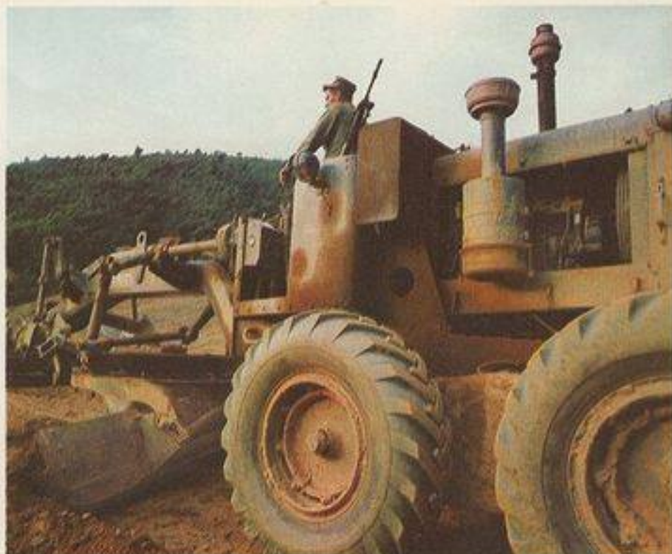
Rifles close at hand, a SeaBee operates a Galion motor grader on an MCB-9 excavation project by the I Corps.
