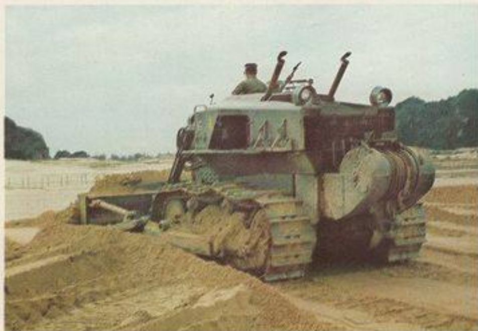
Under SeaBee operation an Eimco bulldozer levels sand dunes along the South China Sea near Da Nang for enlargement of a POW compound.
